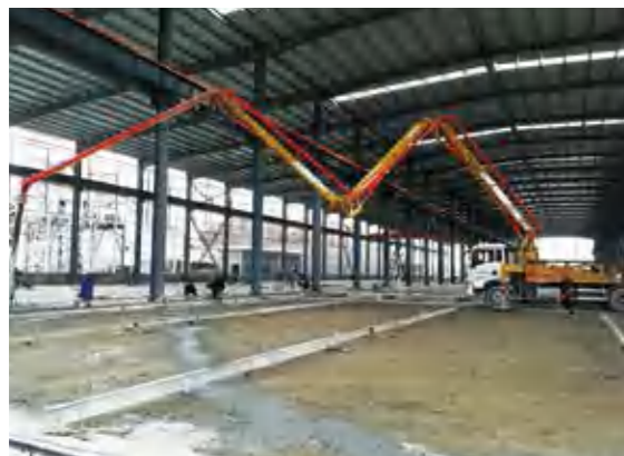
30米泵车厂房内施工 (30米泵车厂房小试牛刀) HB30K boom pump is trying its hand at the workshop.
