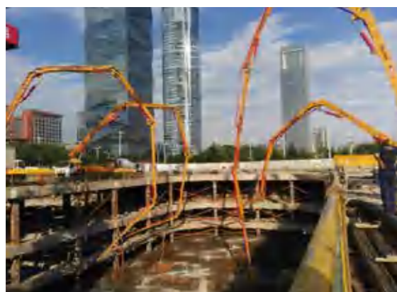
四蛟龙齐助华新城建设 Four boom pumps are cooperating like dragons in Nanjing Huaxincheng Construction.
